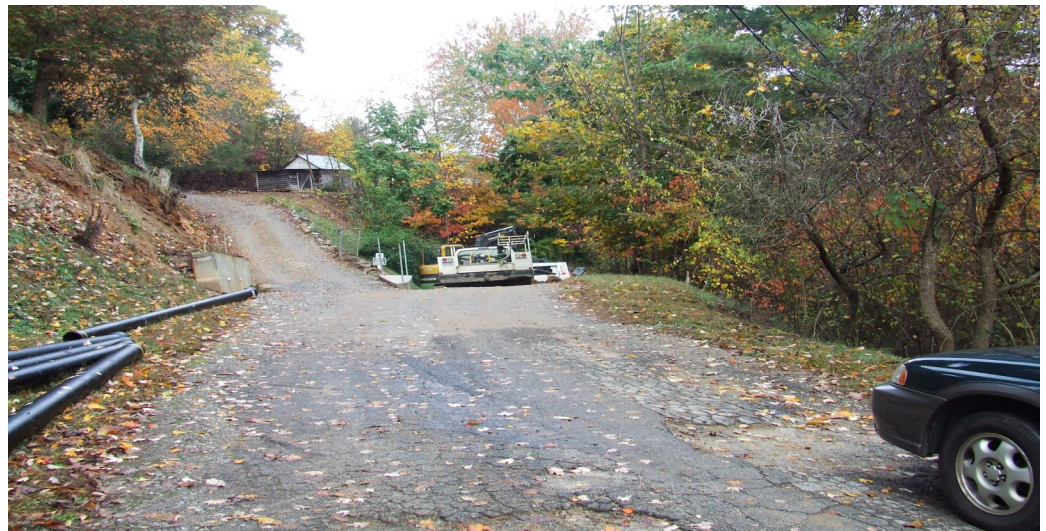
Pipe being laid on the steep drive leading up to Viewmont Acres.
